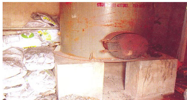
Heat generating system
